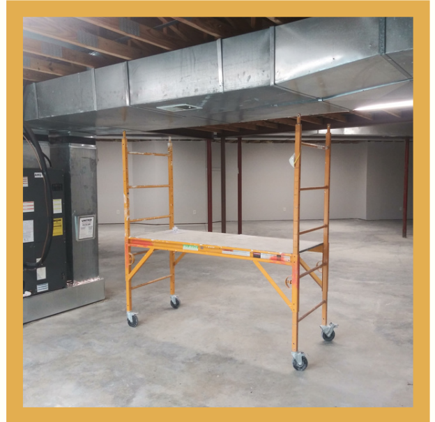
Construction has started on the basement. This picture shows furnace units before they were moved to make space for group therapy
