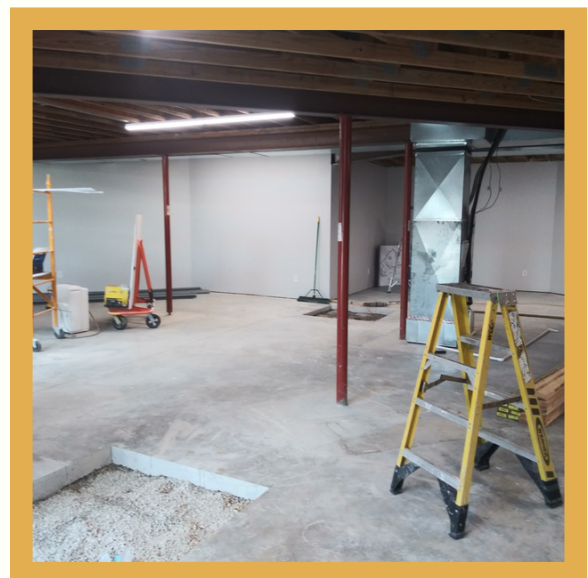
The furnace units have been moved and plumbing is being updated for the teaching kitchen and additional bathroom.
